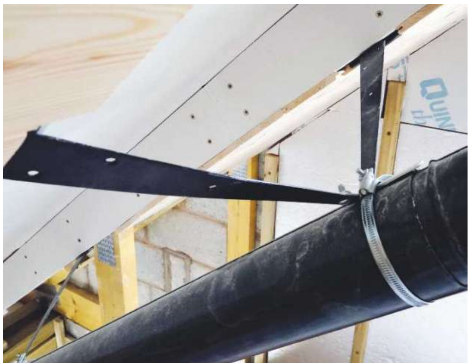
These standard Japanned 'T' hinges were ideal for holding the flue pipe in place
